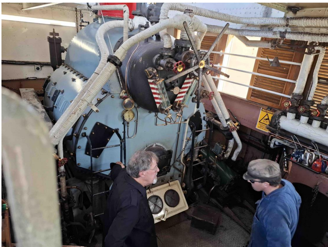
The Yarrow boiler of the Waimarie.
